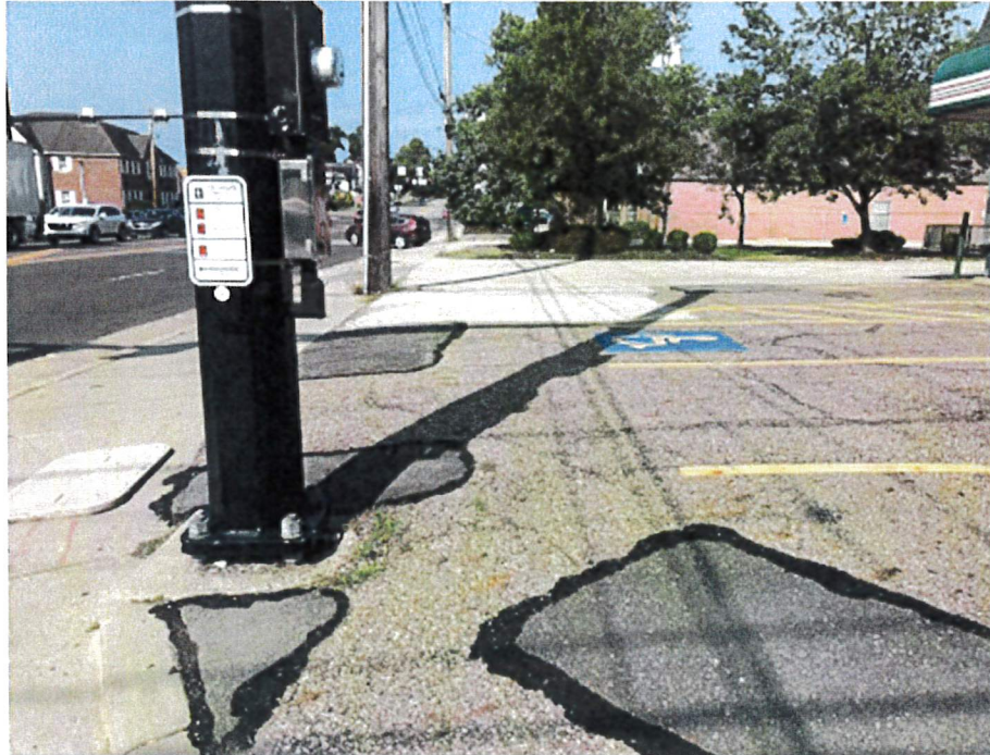
Photograph 3 – View from near station 117+40 facing in a westerly direction showing the Parcel 8T area; a nominal cost to cure has been provided for asphalt resealing in this area to remove existing parking striping
