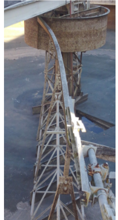
Primary Clarifier #2's 30 foot long skimmer/scrapper arm bent beyond repair in late 2018. The repair from all damage is appx. $.5 million.
