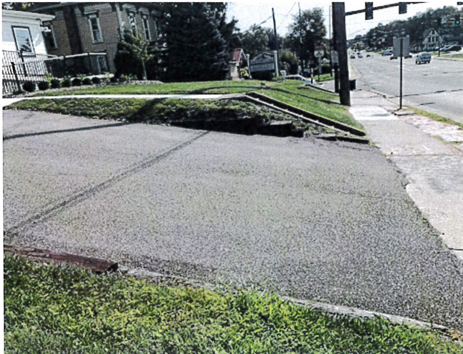
Photograph 2 – View from near station 25+25 facing in an easterly direction showing the Parcel 2T area
